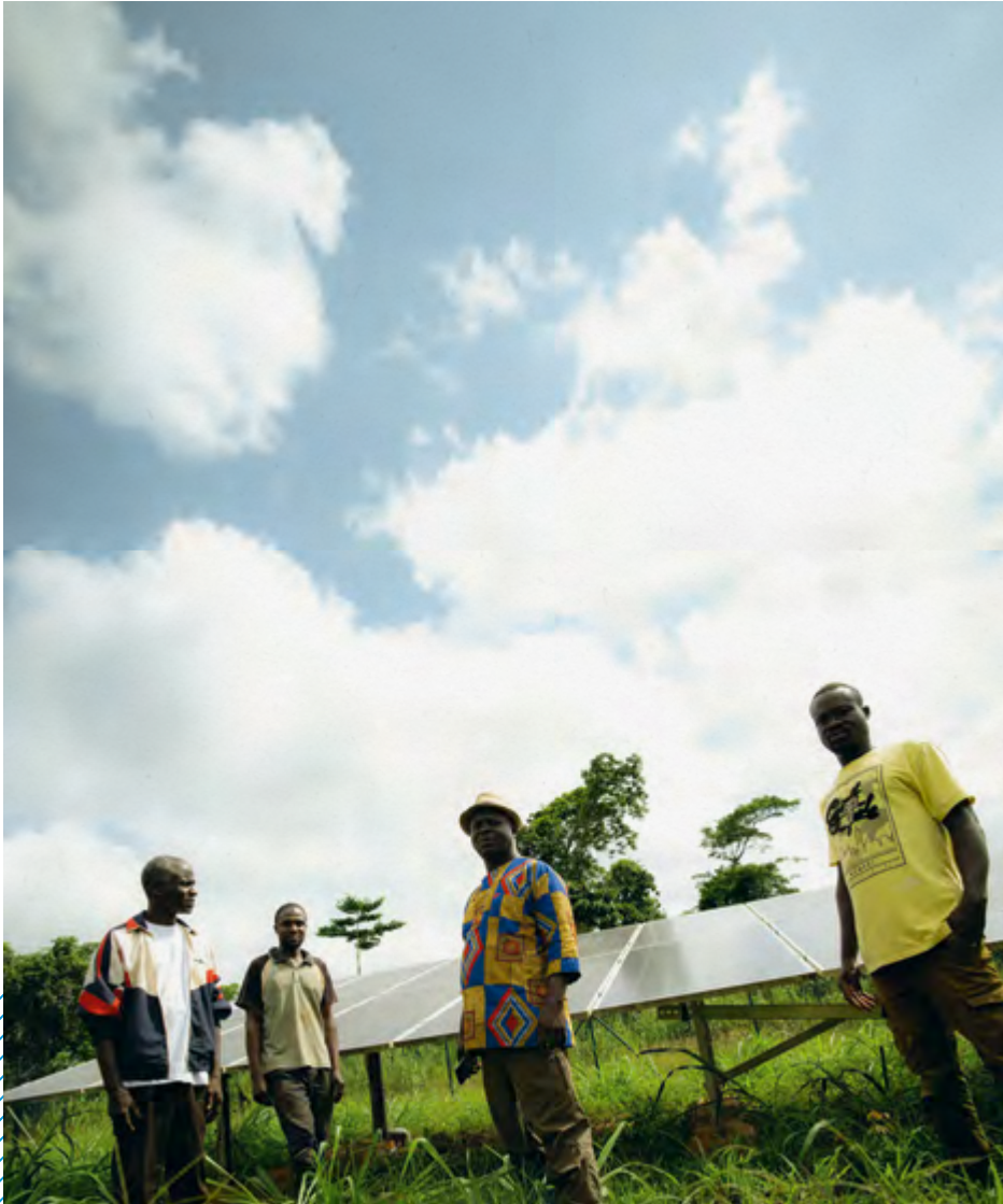
← In Côte d'Ivoire, the village of Dibyko was electrified through the EU's Ecler Ivoire project.
